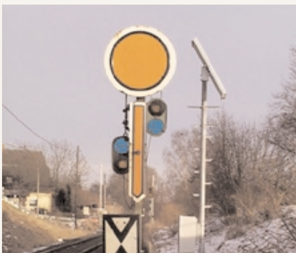
Siemens: Traditional semaphore railway signal illuminated at night with LEDs powered by a solar unit
