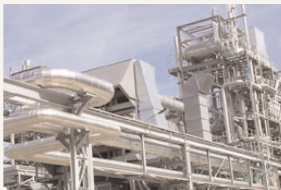
Solvay: Co-generation plant at Jemeppe, Belgium
